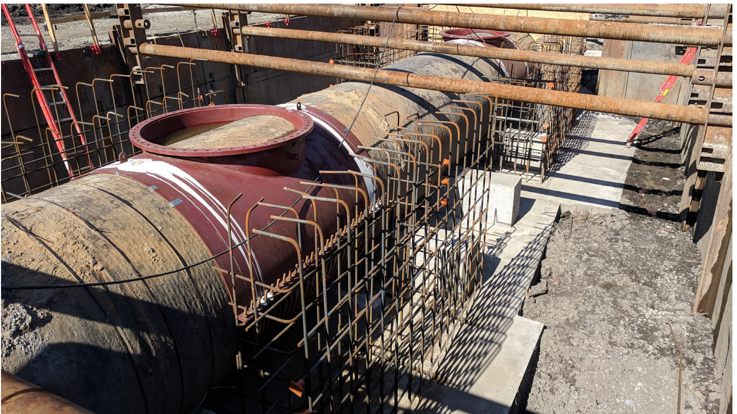
Construction on the Christina River Force Main that conveys wastewater to the Wilmington Water Pollution Control Facility in DE. Photo credit to Delaware Department of Natural Resources and Environment Control.
