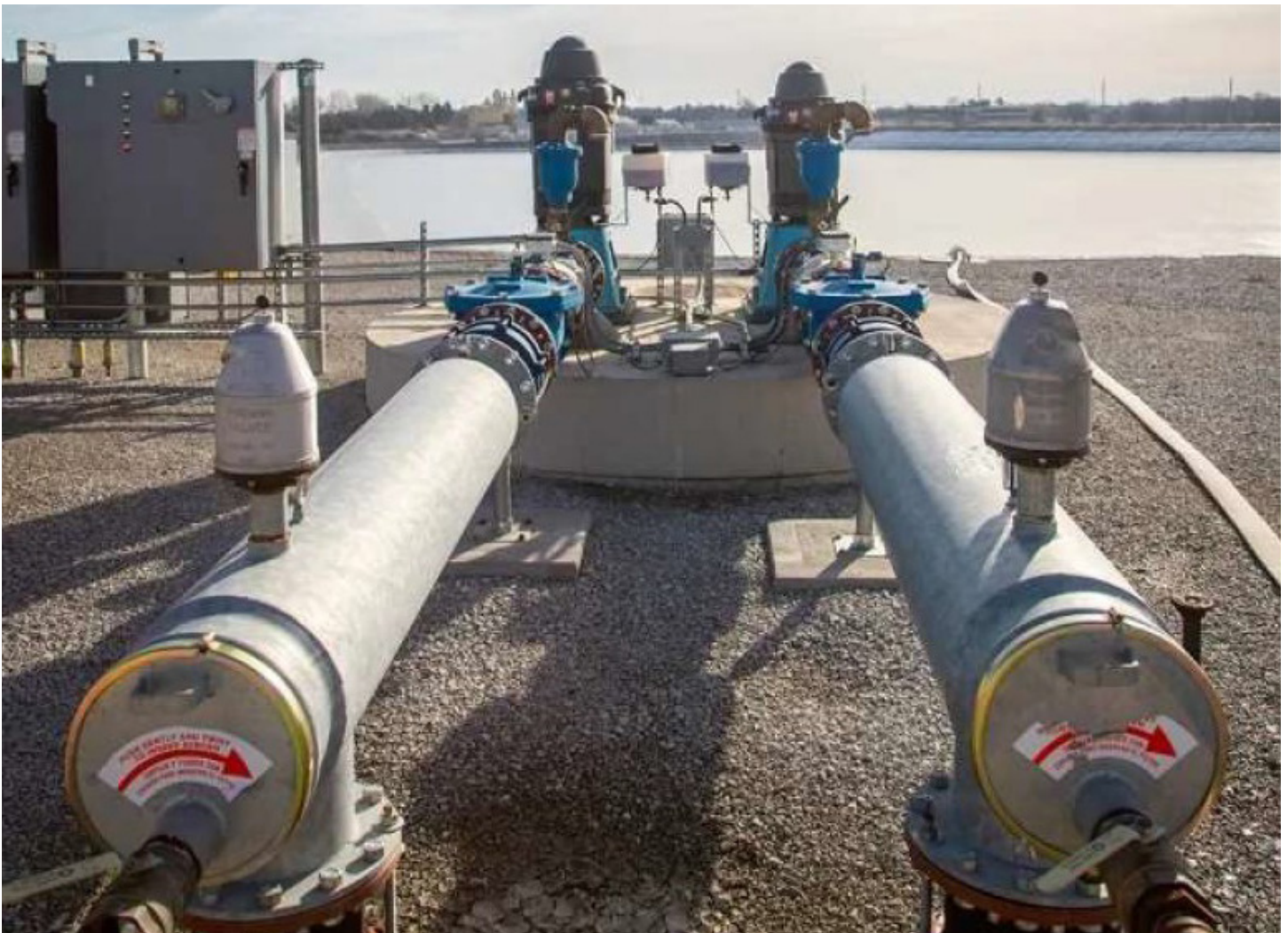
Pumps part of the aquifer storage and restoration project to remove excess nitrogen. Photo credit to City of Hastings, NE.
