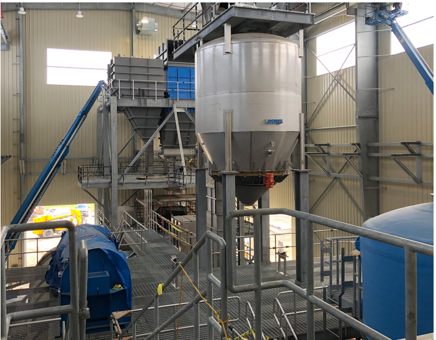
Interior of the biosolids reuse processing facility at the Village Creek Water Reclamation Plant in Fort Worth, TX. Photo Credit: Texas Water Development Board.
