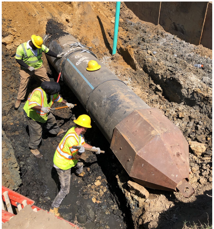
Repairs underway on the Hampton Roads Sanitation District wastewater system in VA. Photo Credit: Virginia Department of Environmental Quality.
