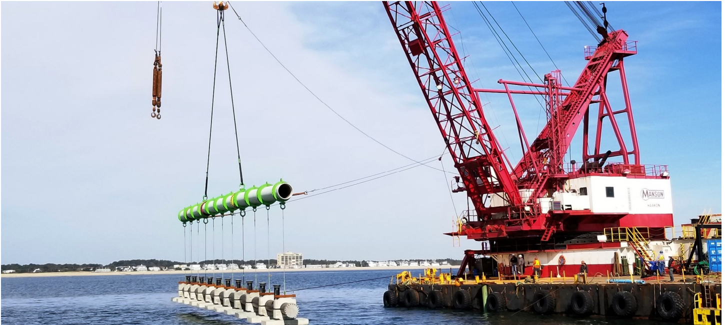
Construction of an ocean outfall pipe as part of upgrades to the local wastewater treatment plant to eliminate discharges to the Lewes and Rehoboth Canal in DE. Photo Credit: Delaware SRF.
