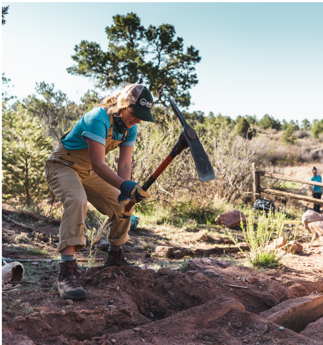
Trail construction in Garden of the Gods, Colorado | Credit: Rocky Mountain Field Institute
