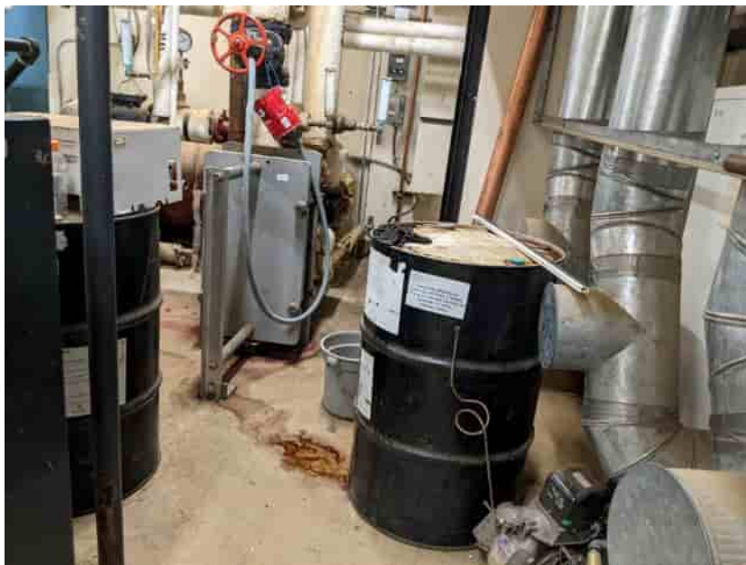
Photo No. 1 – Drums stored inside the boiler room of the water utility portion of the building (HWMU-1). 22 June 2022
