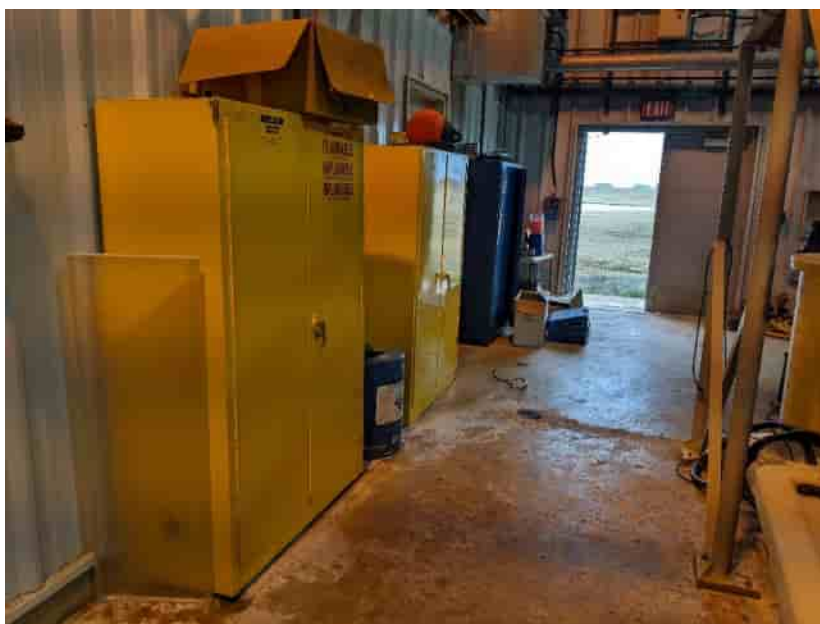
Photo No. 2 – Hazardous product storage in the northwest corner of the Sewage Treatment Plant building (SWMU-1). 23 June 2022
