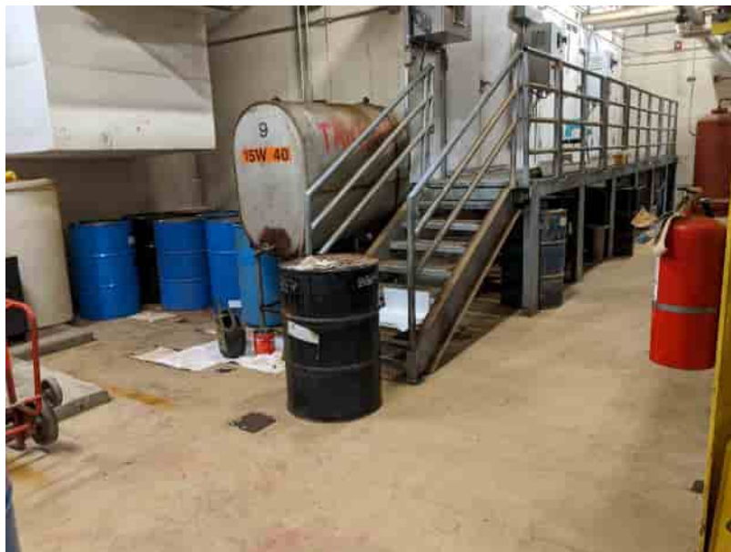
Photo No. 2 – Used oil tank and drum accumulation area within the generator room of the Power Plant. Drums are stored along the wall and under the walking platform (HWMU-1). 22 June 2022
