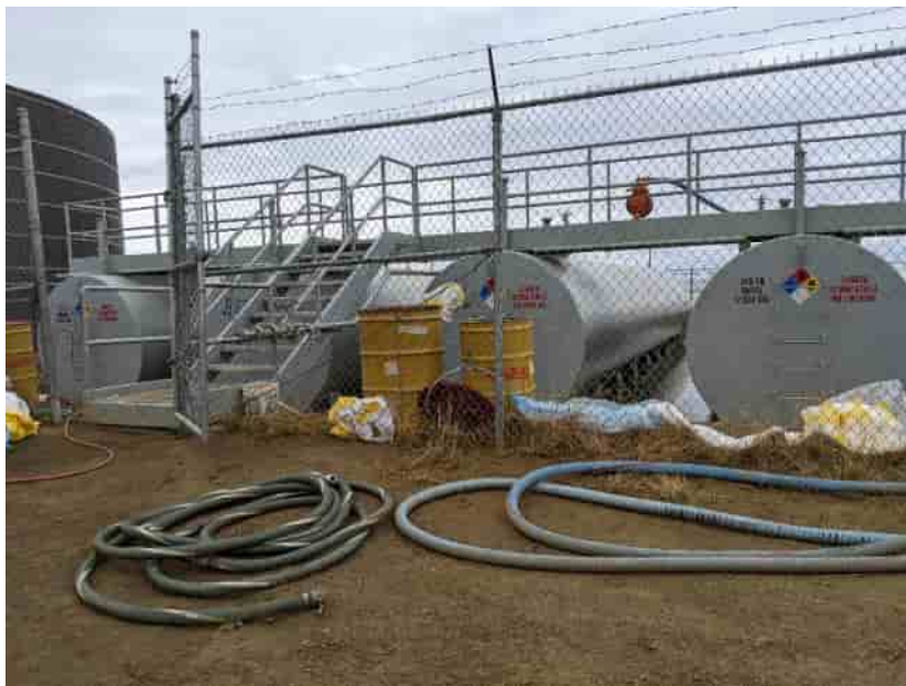
Photo No. 1 – Spill response equipment placed within the fenced area of the Utility Tank Farm (HWMU-4). 22 June 2022
