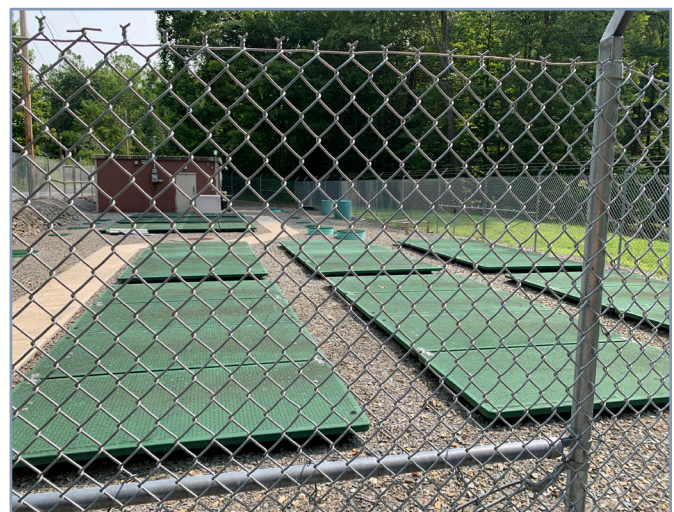
Figure 7. Recirculating treatment system in Winona, West Virginia.
