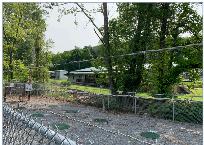
Figure 6. Community septic tank close to homes in Winona, West Virginia.
