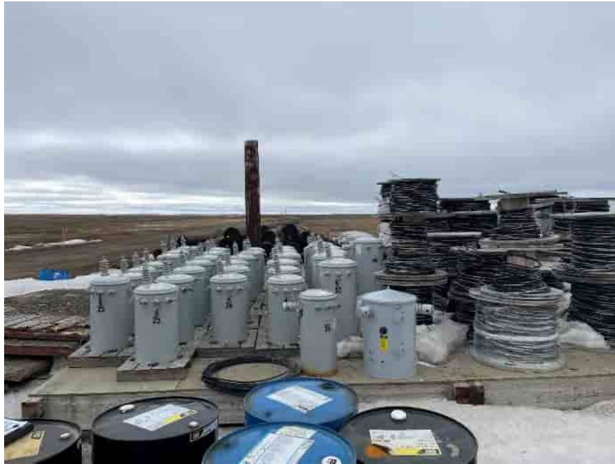
Photo No. 7 – New transformers and wires staged for use. These are not waste; however, the drums in the foreground are waste (HWMU-3). 8 June 2022
