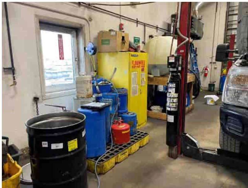
Photo No. 2 – Additional photograph of the interior of the USDW and HEMF building, with wastes and products actively being used and stored on containment pallets (HWMU-1). 8 June 2022
