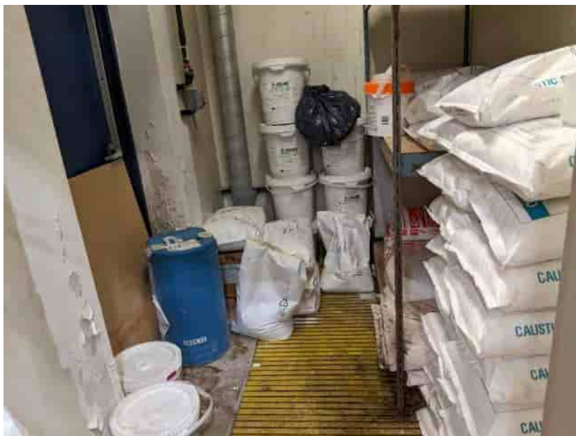
Photo No. 1 – Chemical closet within SWMU-1, the Sewage Treatment Plant building. 3 August 2022
