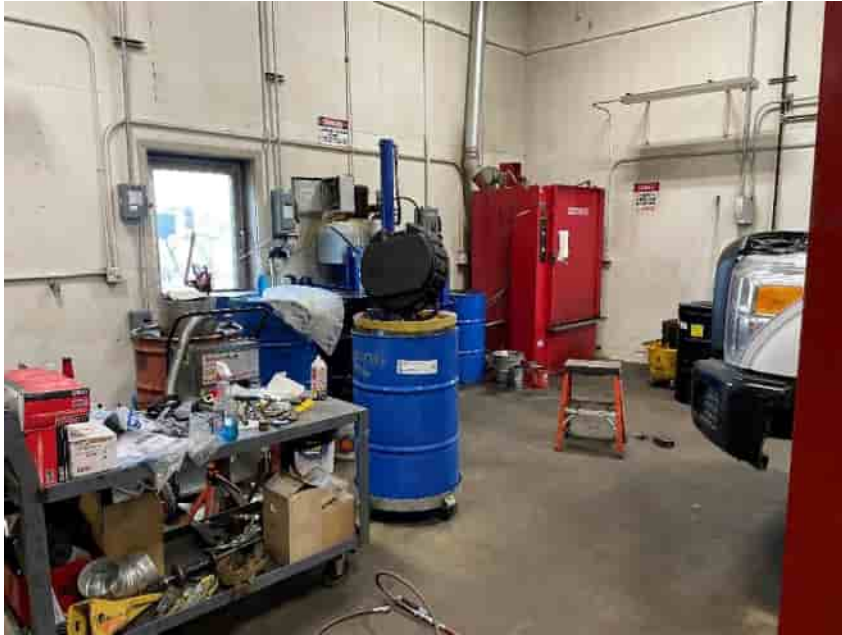
Photo No. 3 – Parts washer in the back corner of the HWMU-1. 8 June 2022
