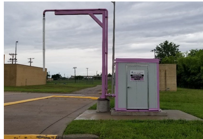
Fill station for dust control
