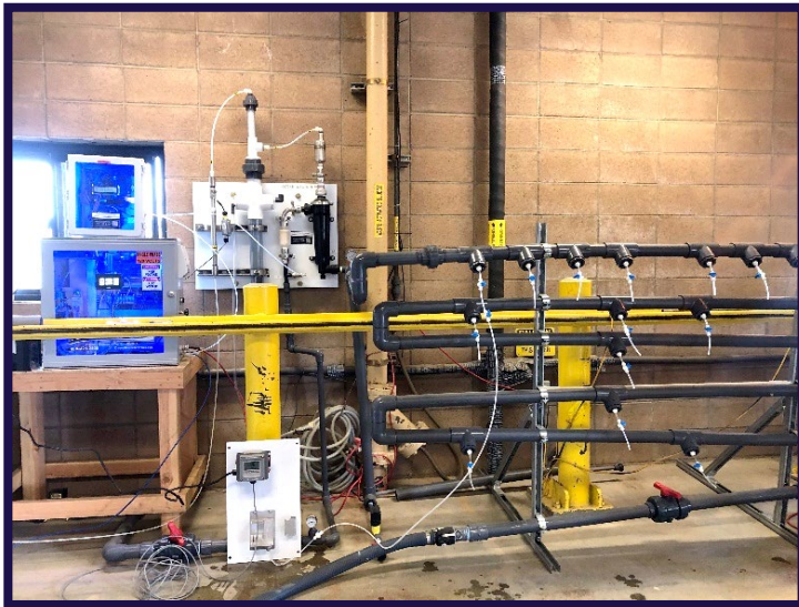
Pilot-scale plug flow ozone contactor system
