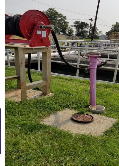
Reclaimed water hydrant for WWTP washdown
