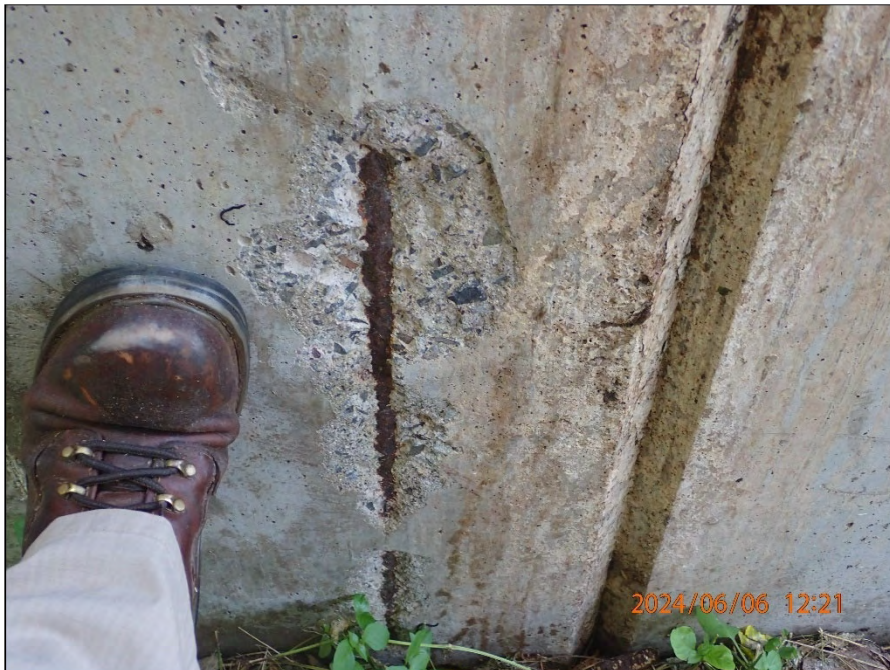
Photograph 14. One spot of Middle Tank's wall had weathered down to the re-bar.
