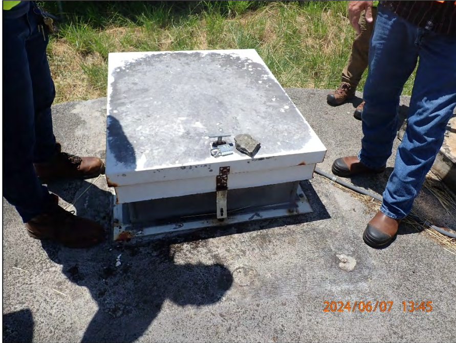
Photograph 17. The access hatch lock was broken as operators attempted to open it.
