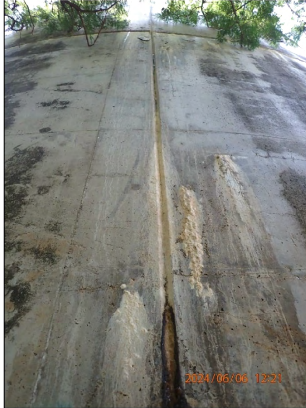
Photograph 13. The concrete tank was leaking and had spalling.
