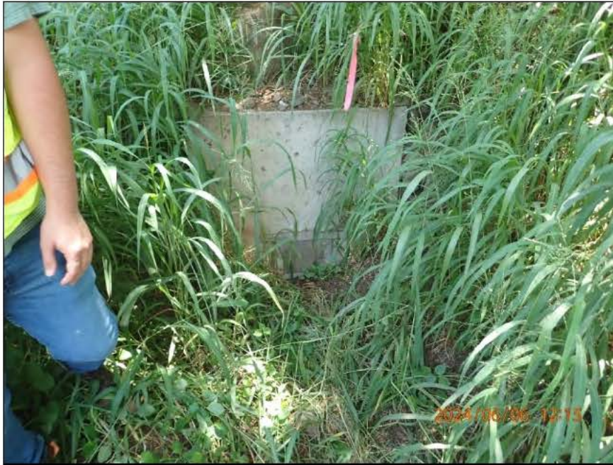
Photograph 11. Middle Tank's overflow flush with the ground and vegetation surrounding it made is more susceptible to potential flooding.
