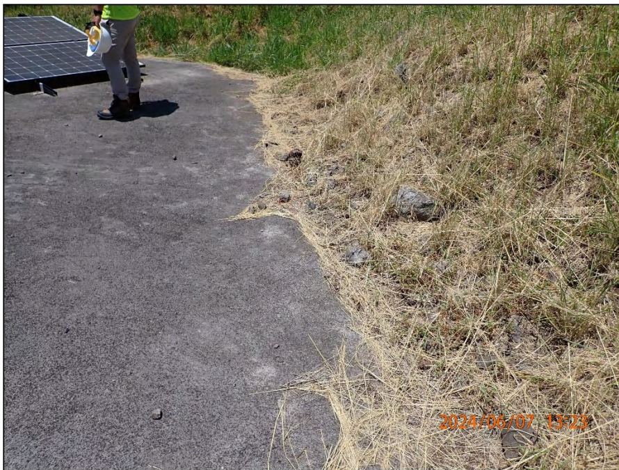
Photograph 16. The hillside was partially burying the North Tank.
