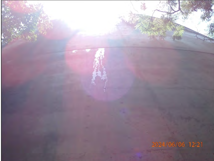
Photograph 15. Middle Tank was leaking water halfway up.
