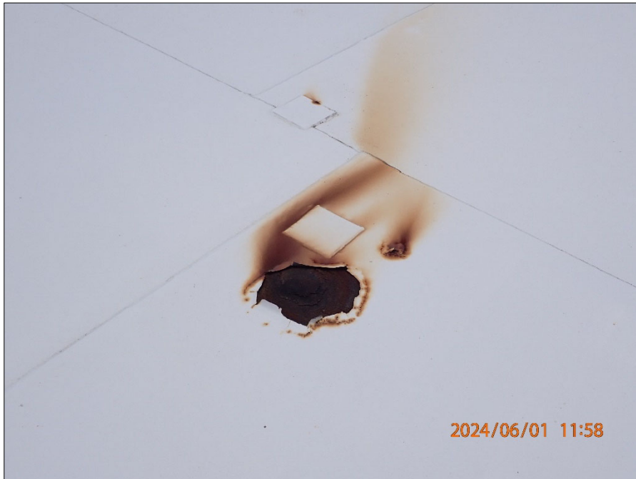
Photograph 12. JBPHH Date/Time Stamp is inaccurate. P6010040.JPG Description: [REDACTED]. Corrosion area on roof.
