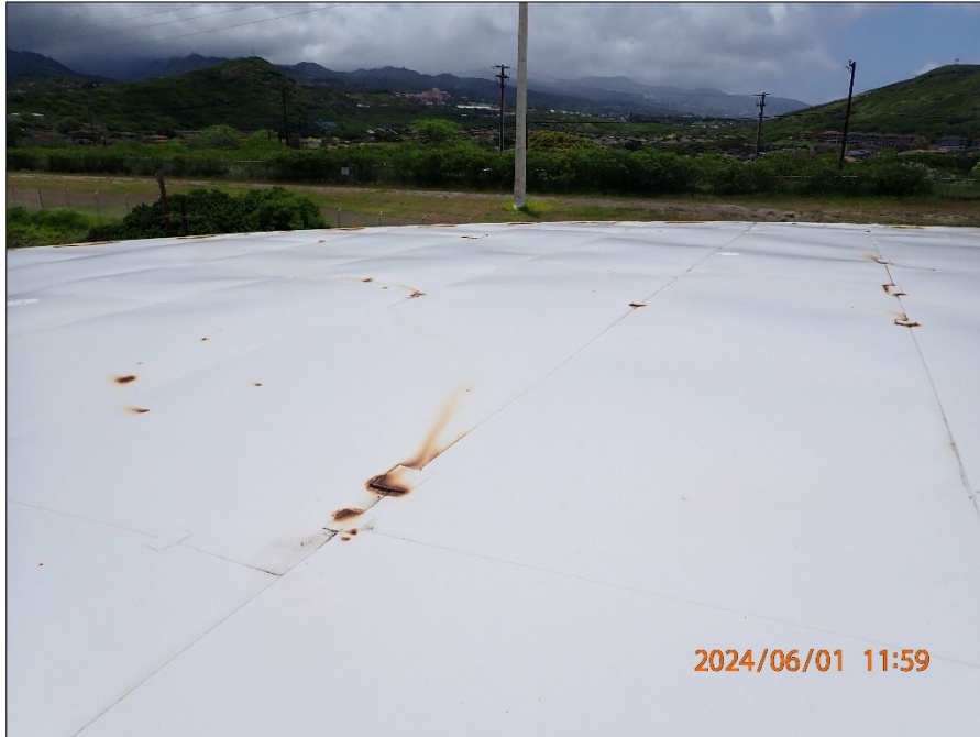
Photograph 11. JBPHH Date/Time Stamp is inaccurate. P6010043.JPG Description: [REDACTED]. Corrosion areas scattered over the light colored roof.
