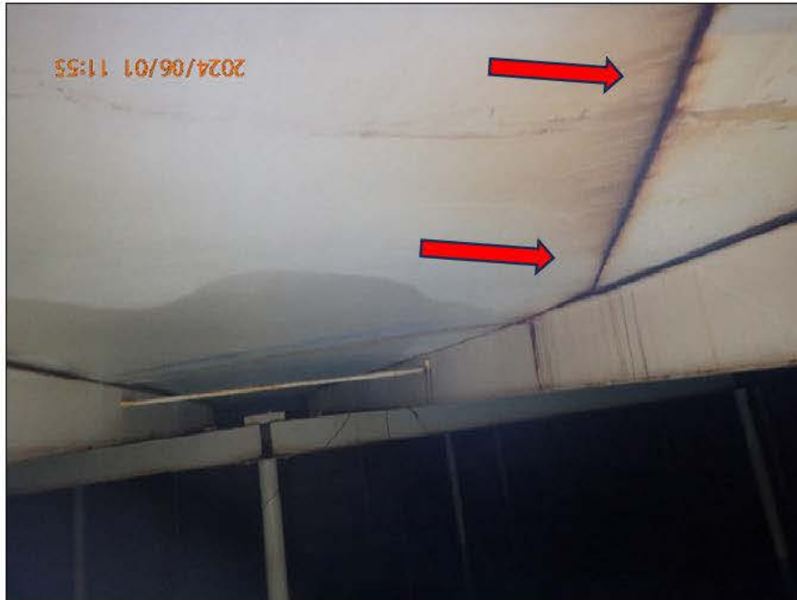
Photograph 9. JBPHH Date/Time Stamp is inaccurate. P6010035.JPG Description: [REDACTED] Corrosion at the joints of the roof interior (callout arrows).
