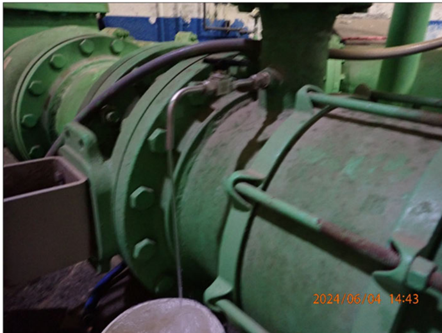
Photograph 52. JBPHH 6/4/2024 14:43 P6040045.JPG Description: Sample location for Sample 006 Red Hill Shaft sample pre-chlorine sample point.
