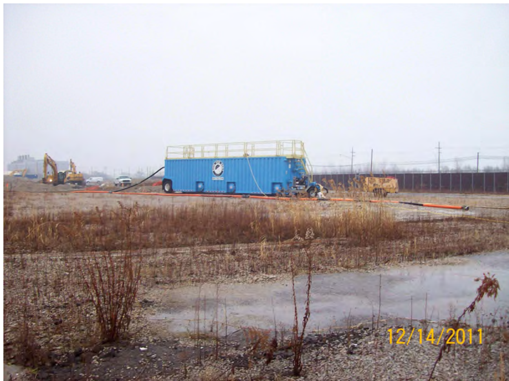
Water filtration & conveyance (view – Northeast)
