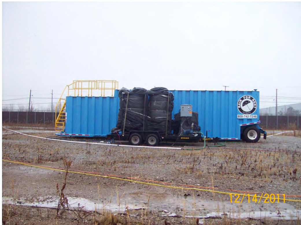
Water Treatment w/freeze protection & Frac Tank Storage (view – East)
