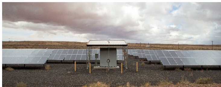
Another view of the site's photovoltaic system. Source: the DOE's Office of Legacy Management
