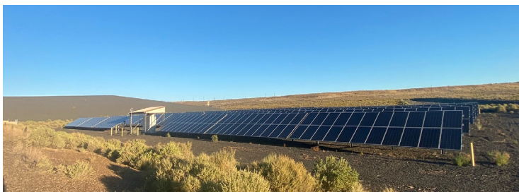
The site's solar photovoltaic system at the disposal cell in Tuba City, Arizona. Source: the DOE's Office of Legacy Management
