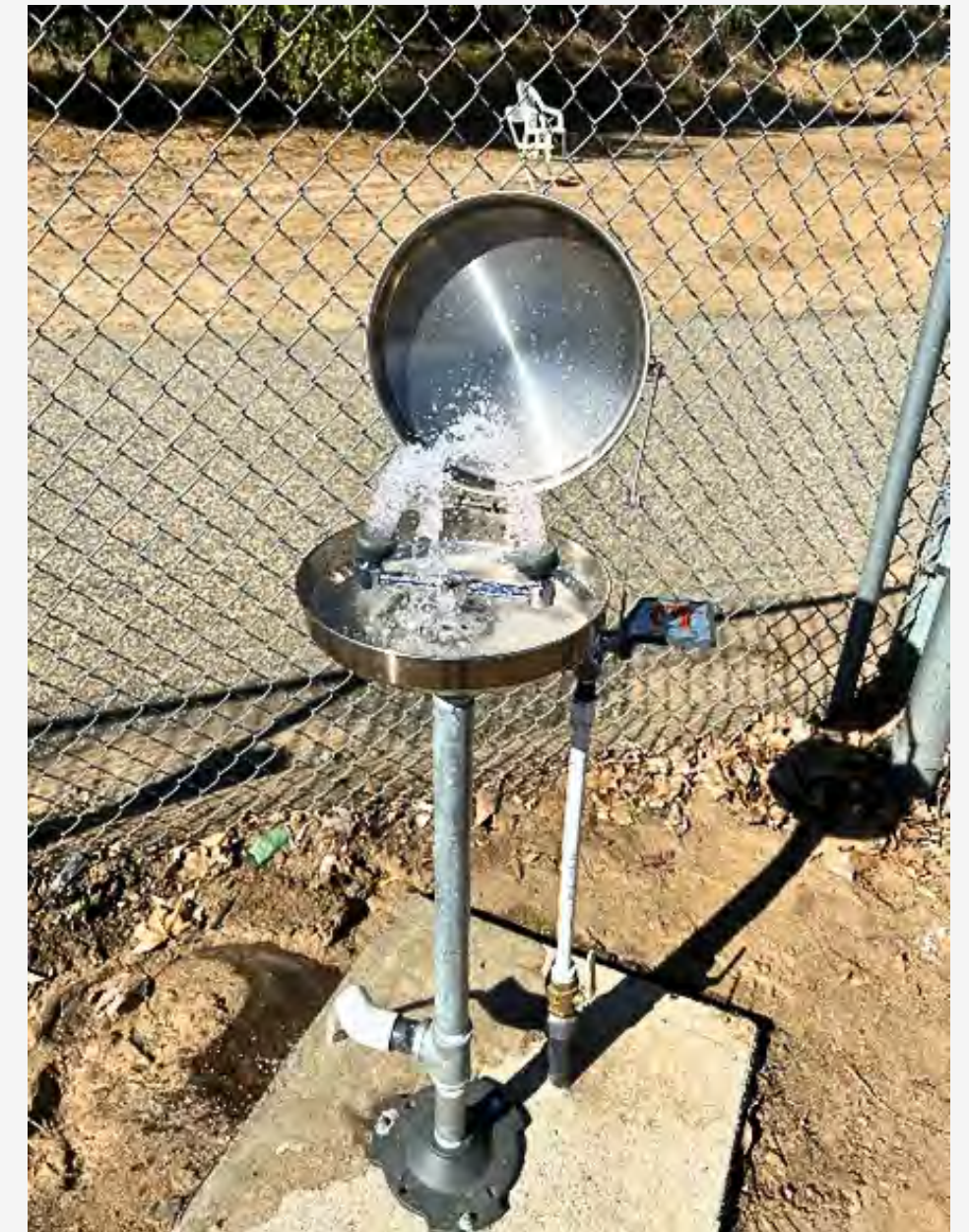
Eyewash Station installed next to the household hazardous waste area
