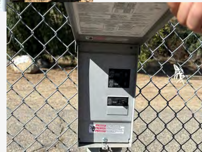
Installed 50 amp sub panel
