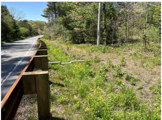
Roadside Swale with Check Dam (Credit: HW)
