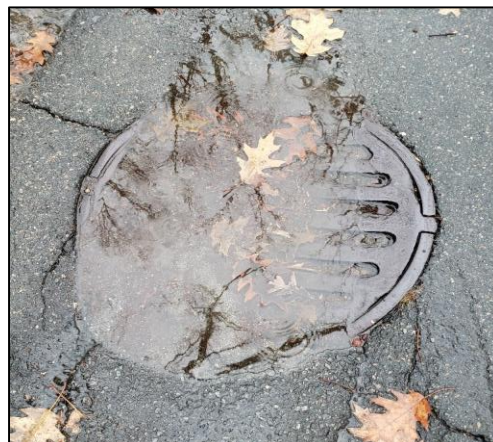
Clogged catch basins can lead to street flooding and release pollutants into receiving waters. Credit: L. Schiffman
