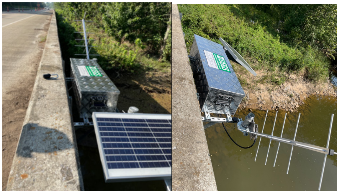
Figure 26. New USGS flow gages on Obion Creek (left) and Mayfield Creek (right).
