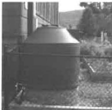
Cistern - Center Pope Elementary School, Easthampton
