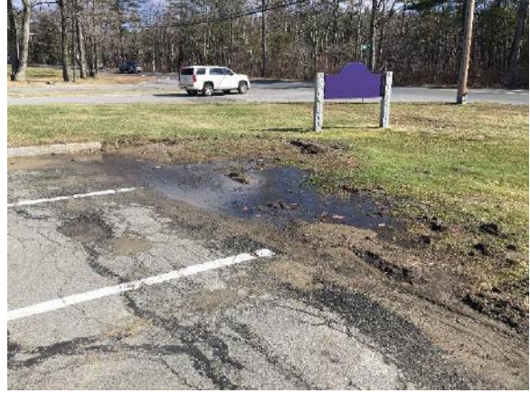
Figure 3. Ponding and Sedimentation near Site
