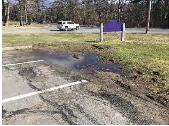
Figure 3. Ponding and Sedimentation near Site
