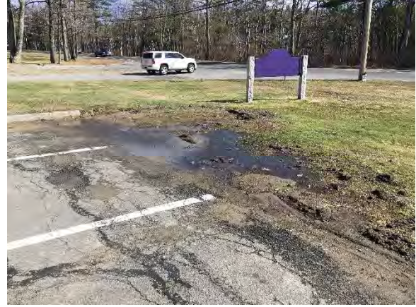
Figure 3. Ponding and Sedimentation near Site
