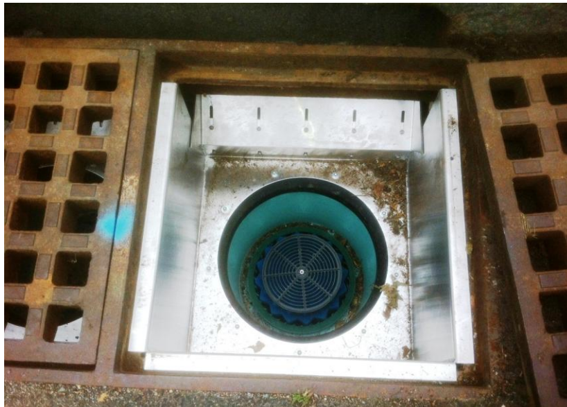
New Storm Drain Filters
