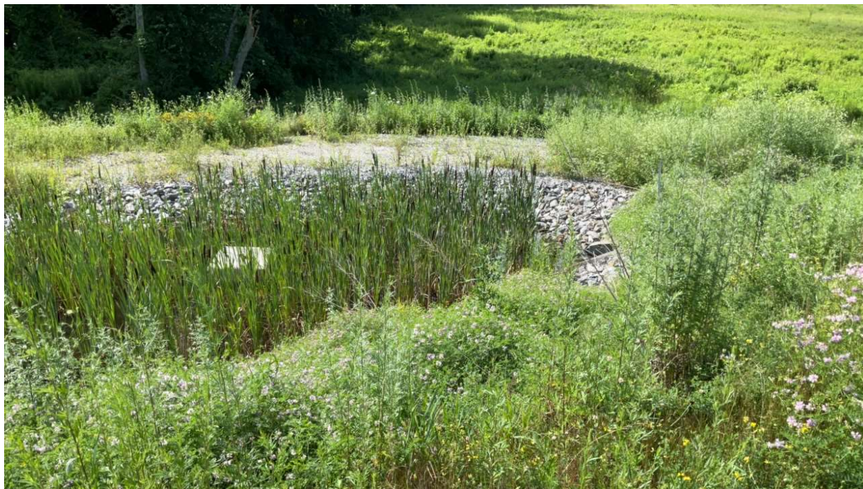
An example of a well-maintained forebay to a treatment facility in Bedford NH, which discharges to the BOWMAN BROOK.
