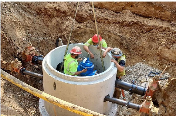
Pressure reducing valve meter pit for the River Road water extension.
