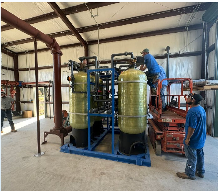
Arsenic removal and sand filter skid.
