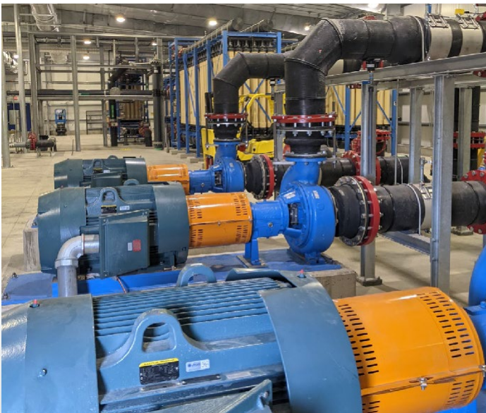
Water treatment plant pumps.
