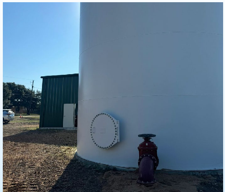
New 50,000-gallon ground storage tank.
