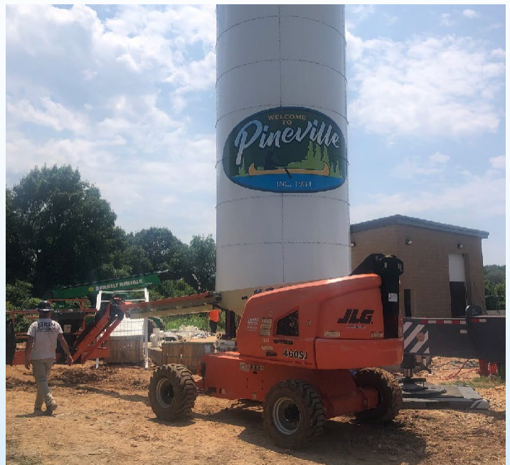
Construction of tower and water treatment plant to house water treatment technology.
