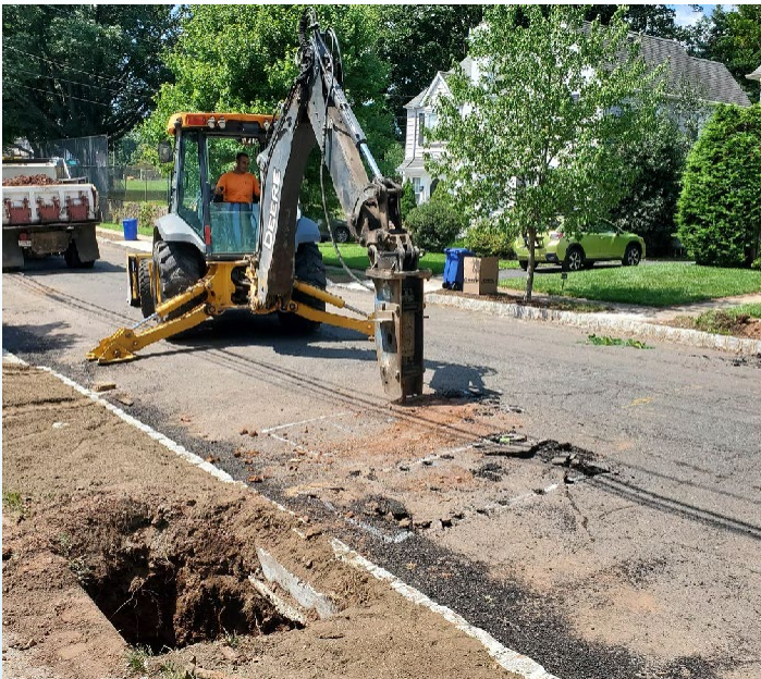
Project consultant oversees the replacement of a lead service line discovered during the first phase of this contract.
