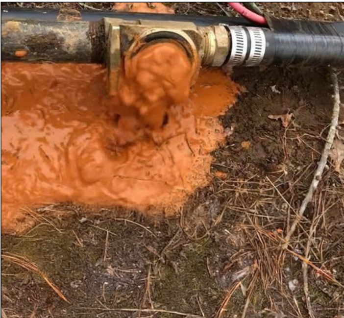
Rockland Oaks discolored water.
