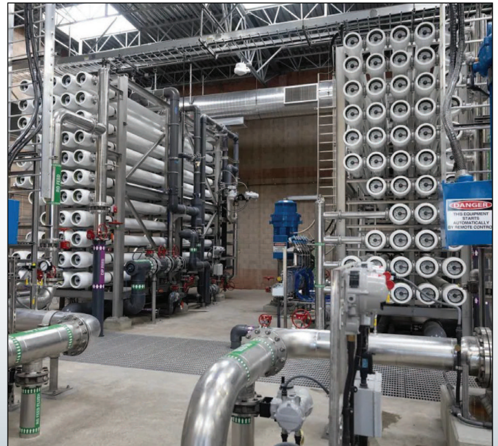
Final reverse osmosis train and booster pump station, used to remove salts and contaminants from drinking water and move treated water through the system.
