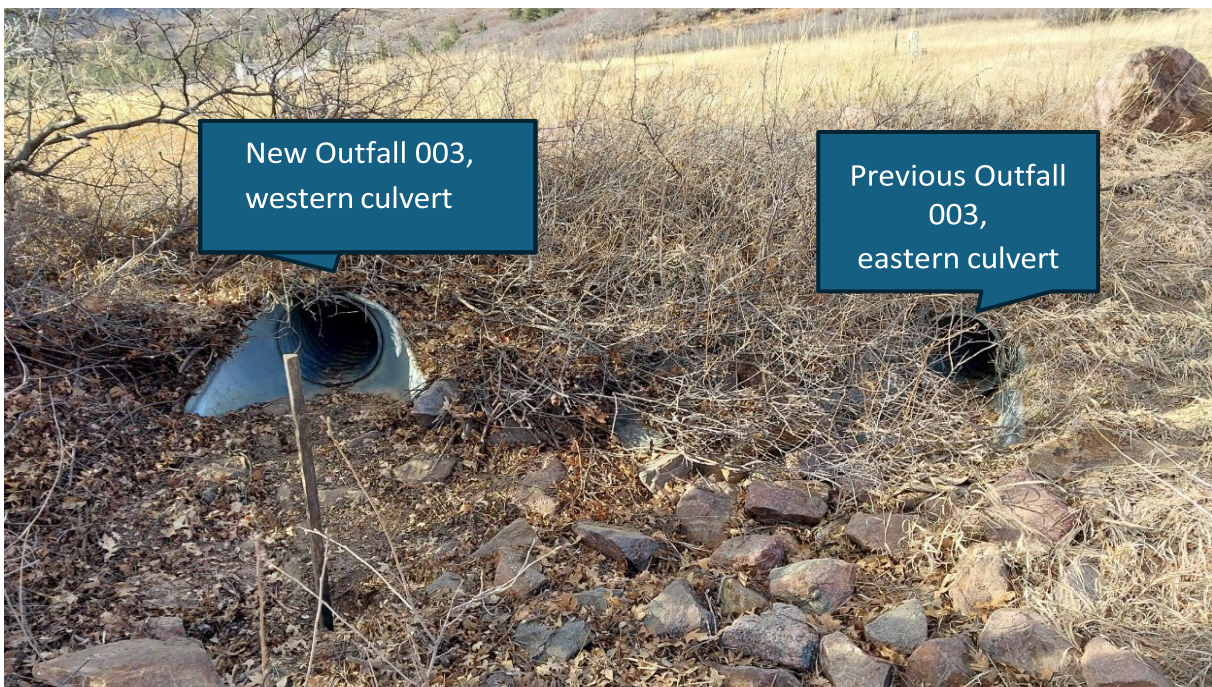
Figure 4. Photo of both previous and new outfall location with vegetation at the western culvert cleared.
