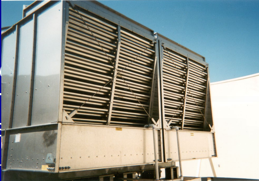
650-ton induced draft CT serving an office complex
