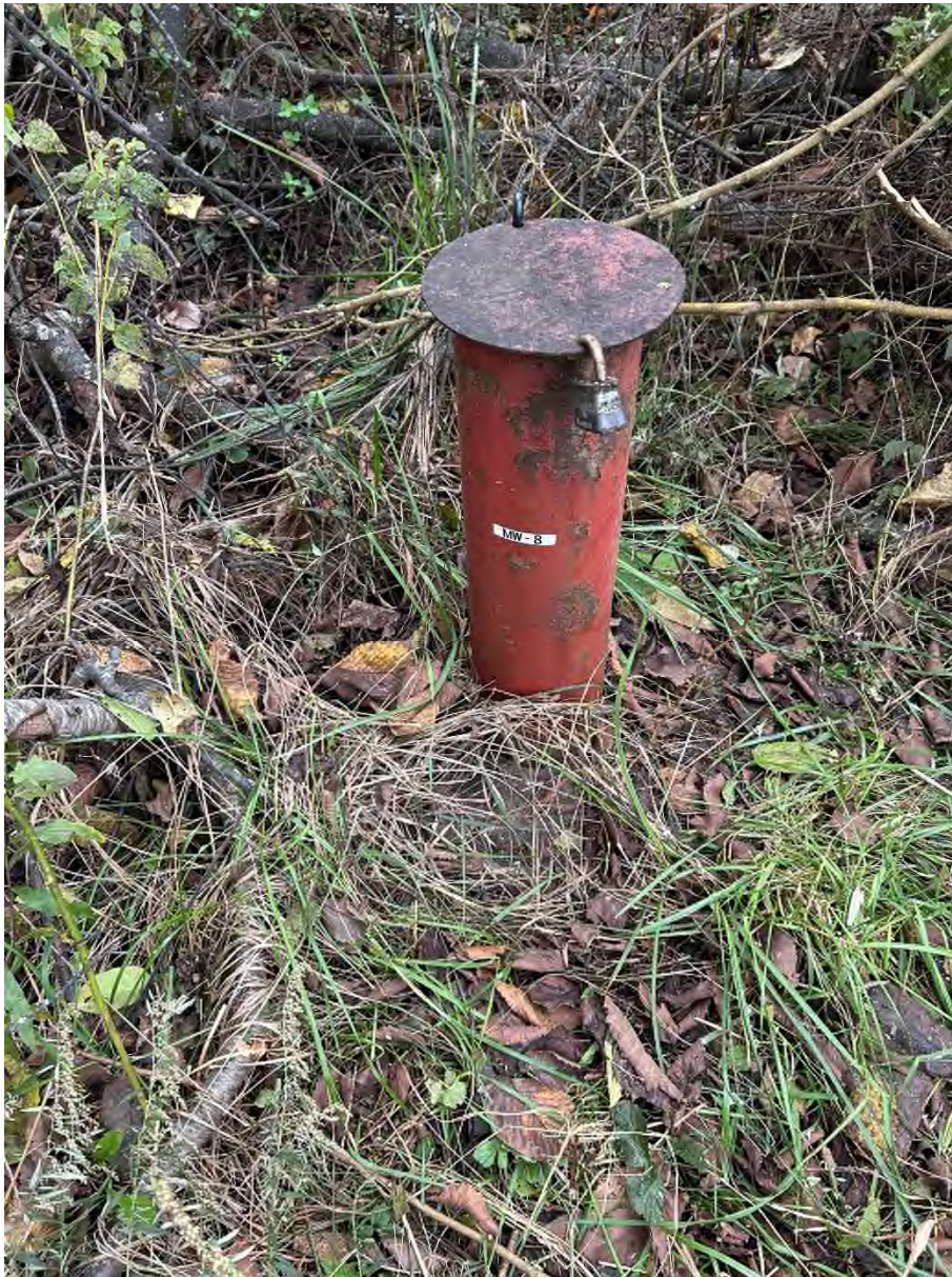
Figure 4: Image of the well MW-8 as seen during the site walk.
