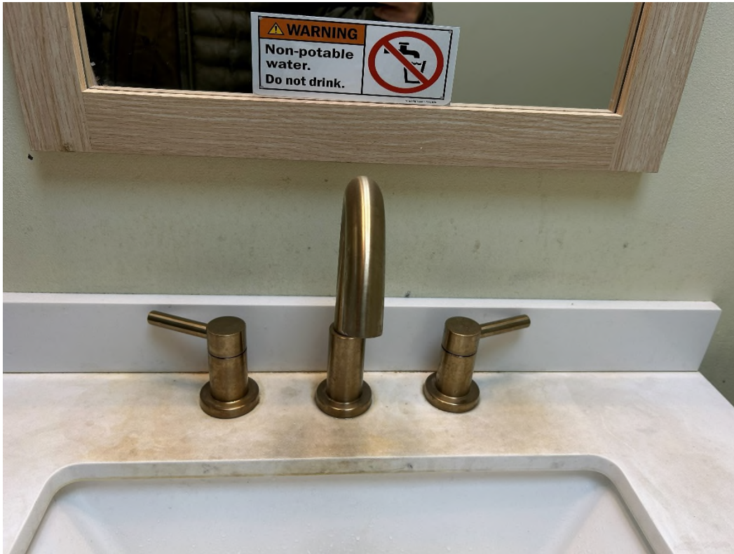
Figure 2: Groundwater use in the facility is limited to non-potable with signs posted accordingly.
