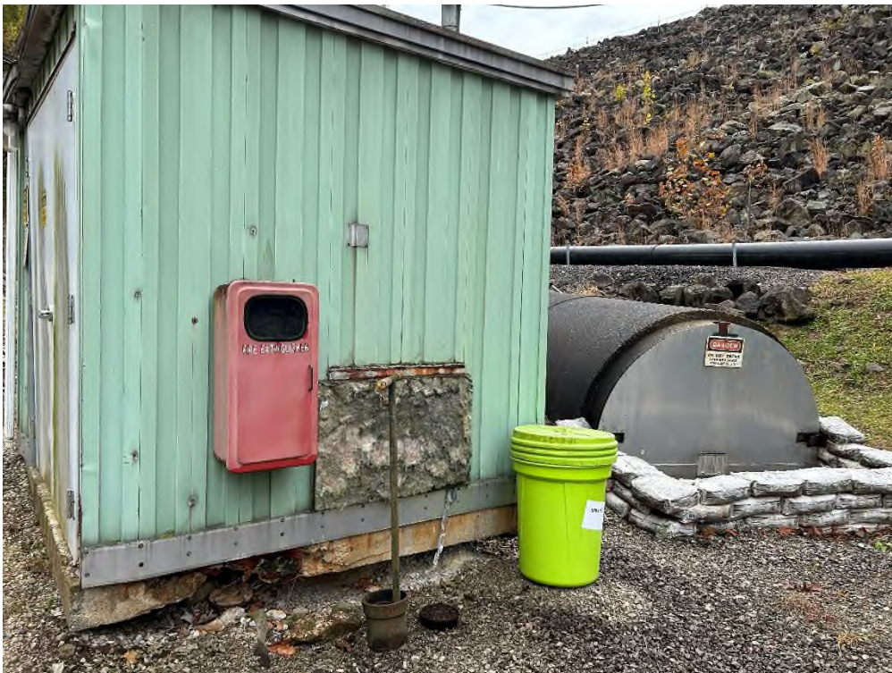
Figure 7: Leachate collection tank and pump housing for the Lower Ward Landfill.
