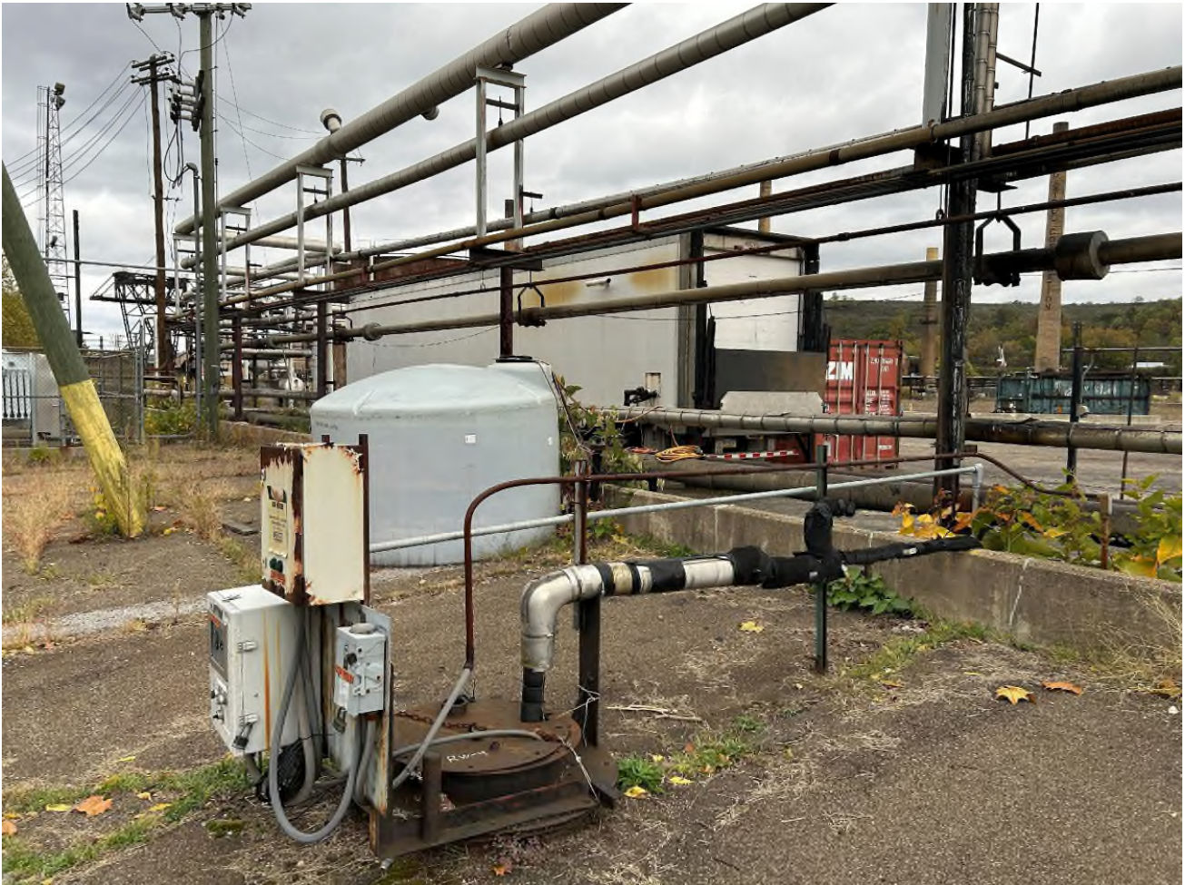
Figure 3: One of the perch groundwater recovery wells (RW-4) with the trailer that houses the standalone groundwater treatment system that became active in April 2021.
