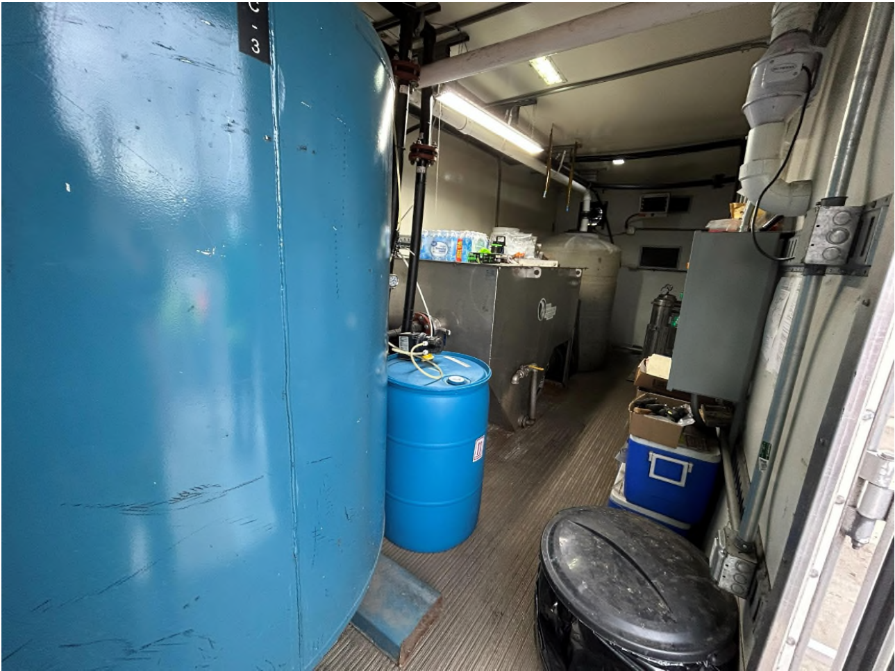
Figure 5: Another image from the inside of the trailer with perched groundwater treatment system components.
