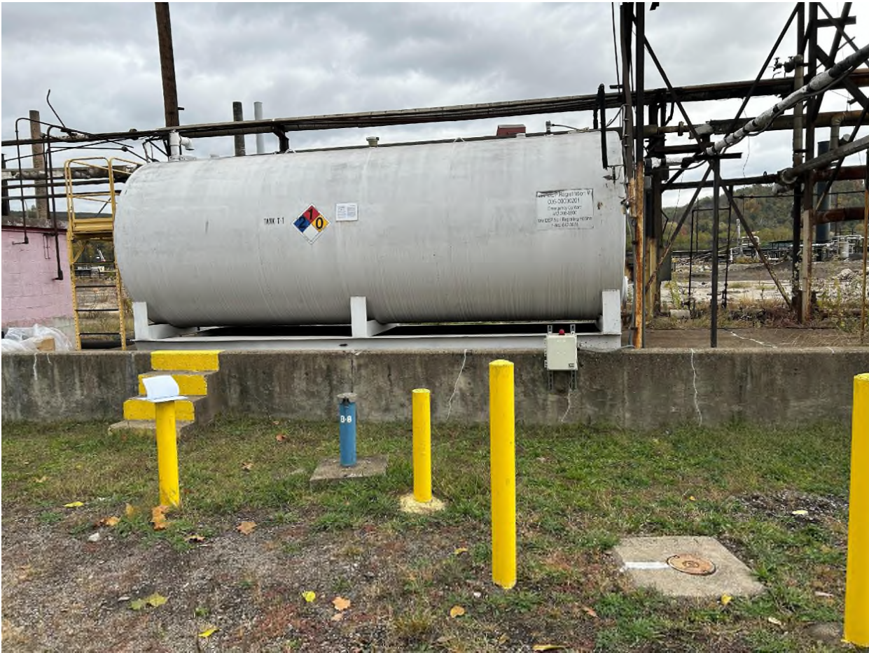
Figure 2: Temporary Storage Tank T-1 for recovered DNAPL before off-site transport and disposal.
