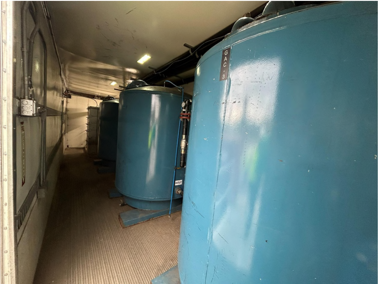
Figure 4: An image showing the inside of the trailer with the groundwater treatment system tanks.
