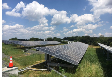
A solar farm in Cinnaminson Township in New Jersey. The solar farm is located on a portion of a former Superfund site that was successfully redeveloped into an alternate energy source. (EPA image)
