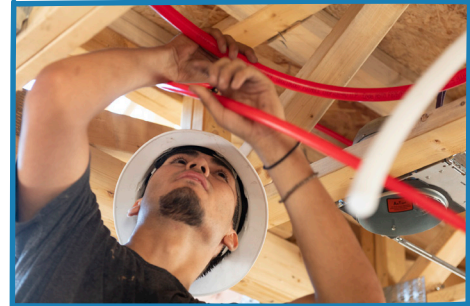
A plumber installing PEX piping for hot water distribution in a new home.
