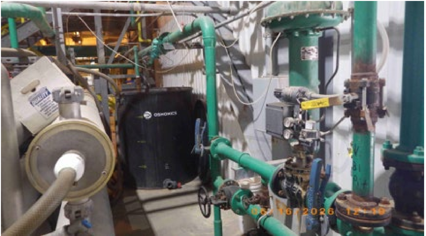
Figure 4 – CO-PF00103 Outfall 001- Cooling Tower 4D
