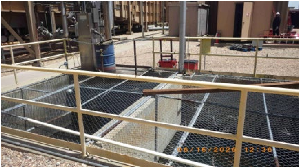
Figure 2 – Brush #1 and 4D Wastewater Treatment Pit
