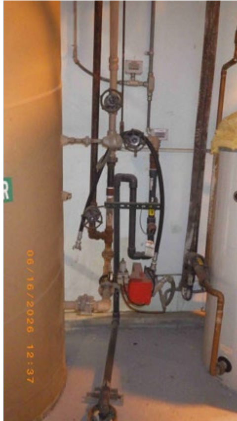
Figure 3 – CO-PF00103 Outfall 001 - Cooling Tower 1
