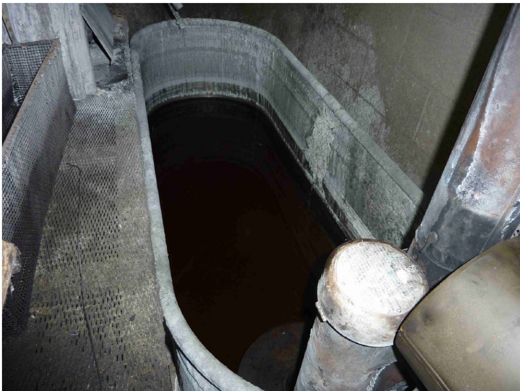
Figure 4 – Evaporative Holding Tank
