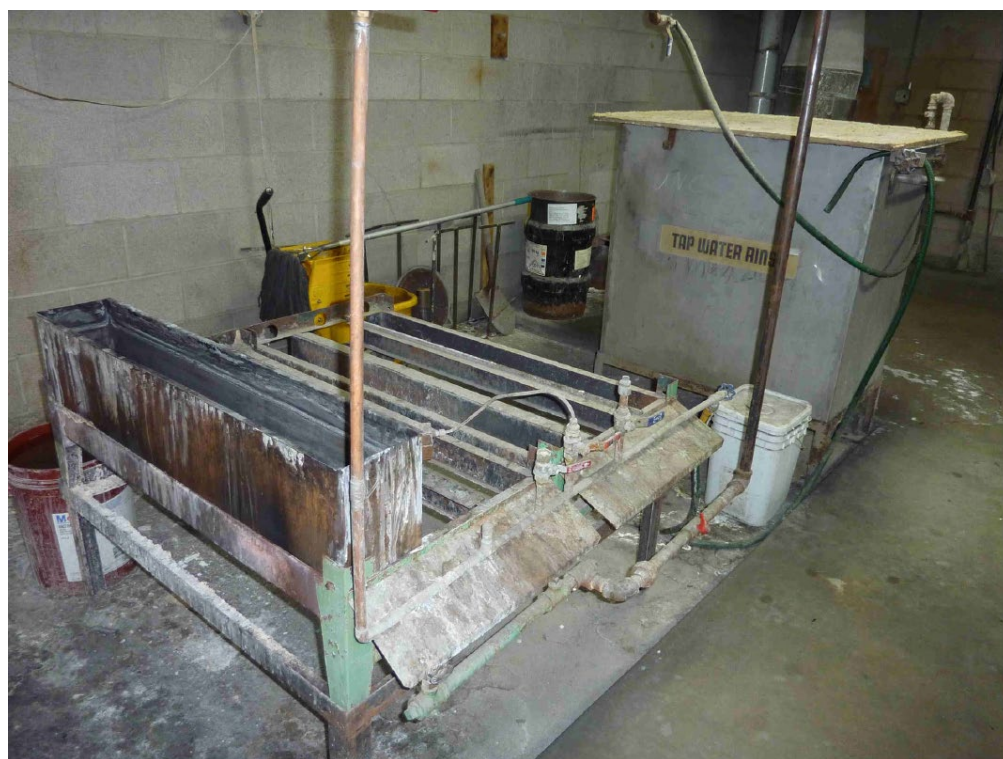
Figure 7 – Case Hardening Process Line
