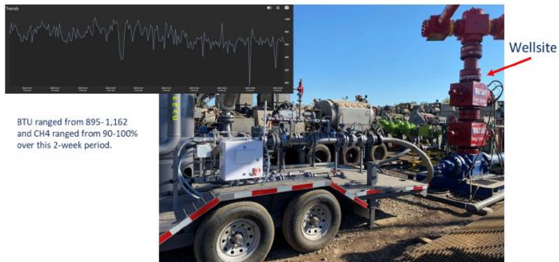
Figure 43: Well Site Example Installation
